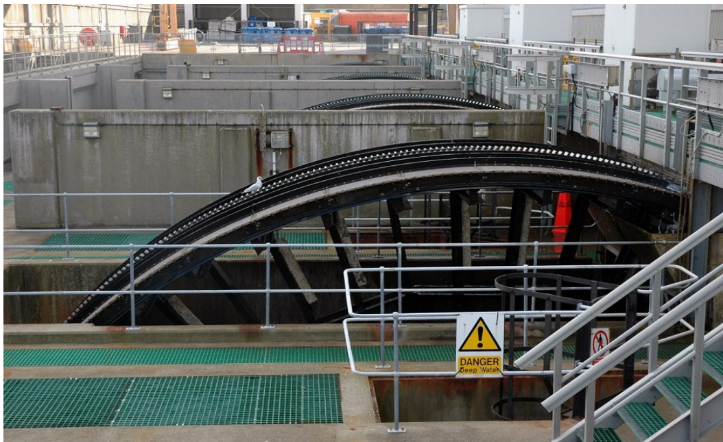
Figure 2.1 The four drum screens at Sizewell B
